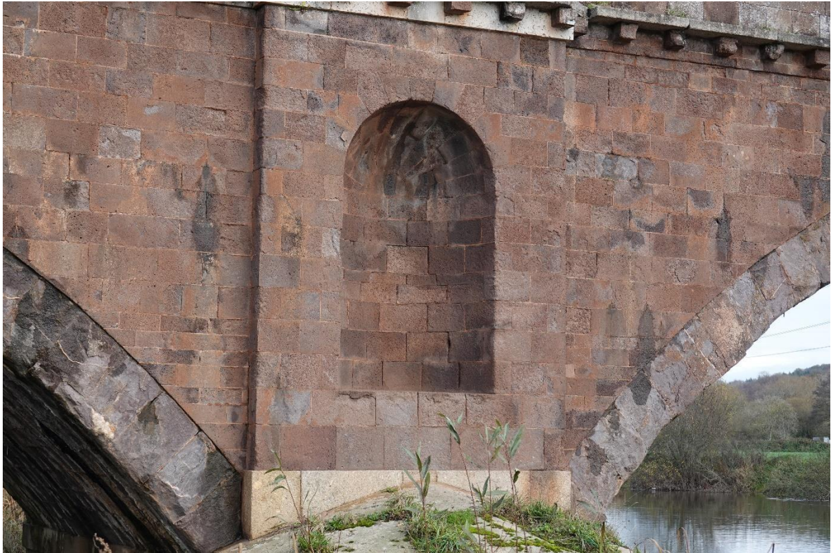
The first thing I noticed on my visit was this crack over the western pier. It looks worthy of note but not a sign of real damage.
