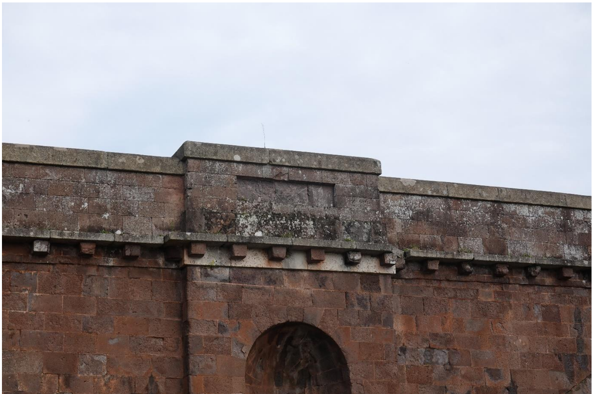
Some of these colour differences are changes due to weathering, others are different stones.
