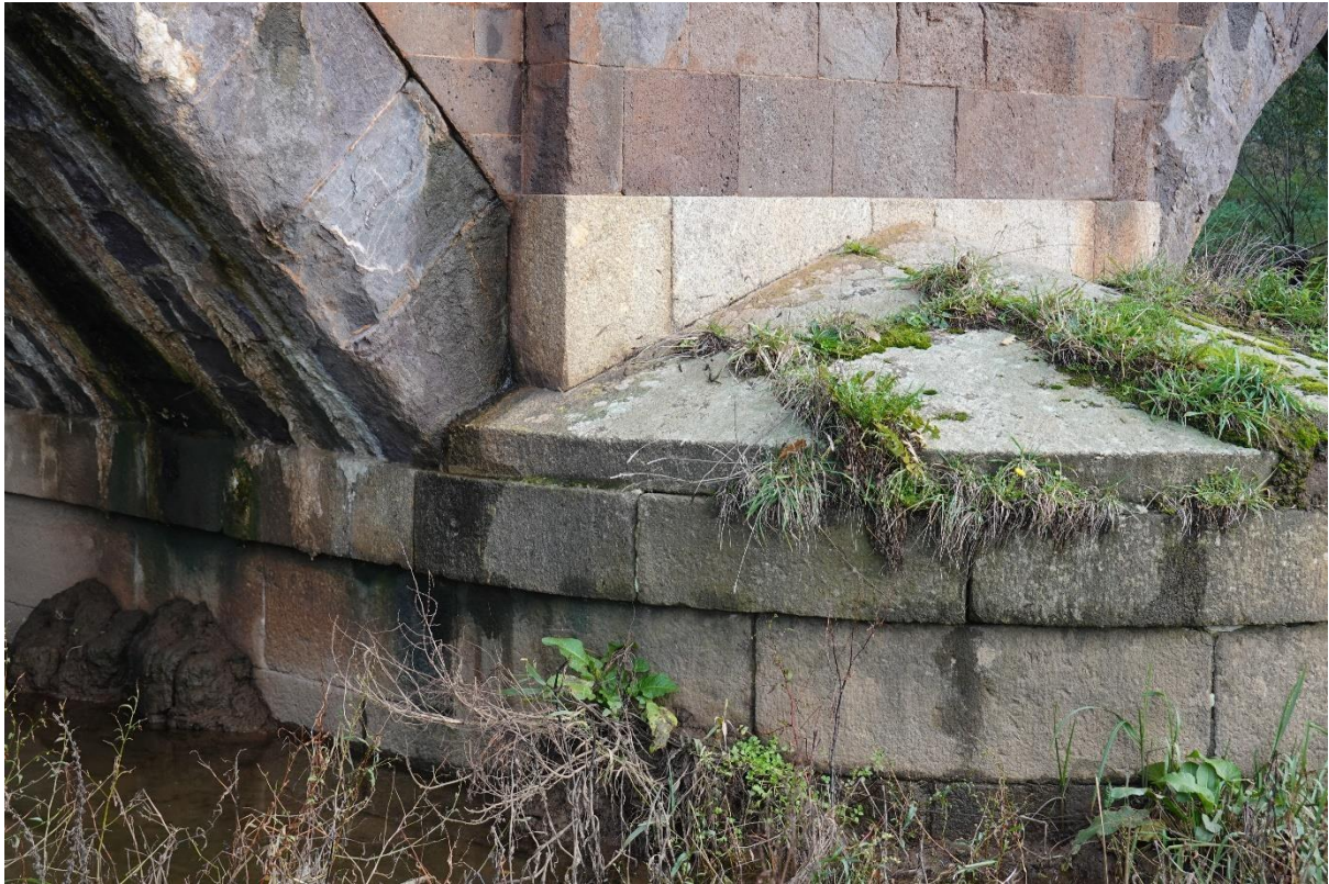
The piers are of granite, the better to resist the effects of the river.
