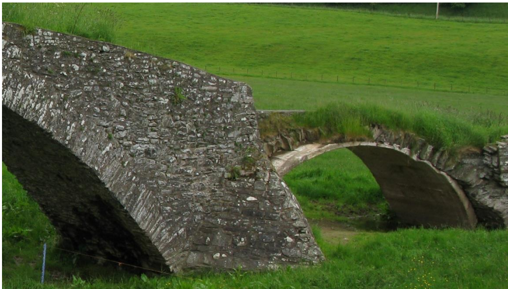
The loss of material also extends to the second flood arch.
