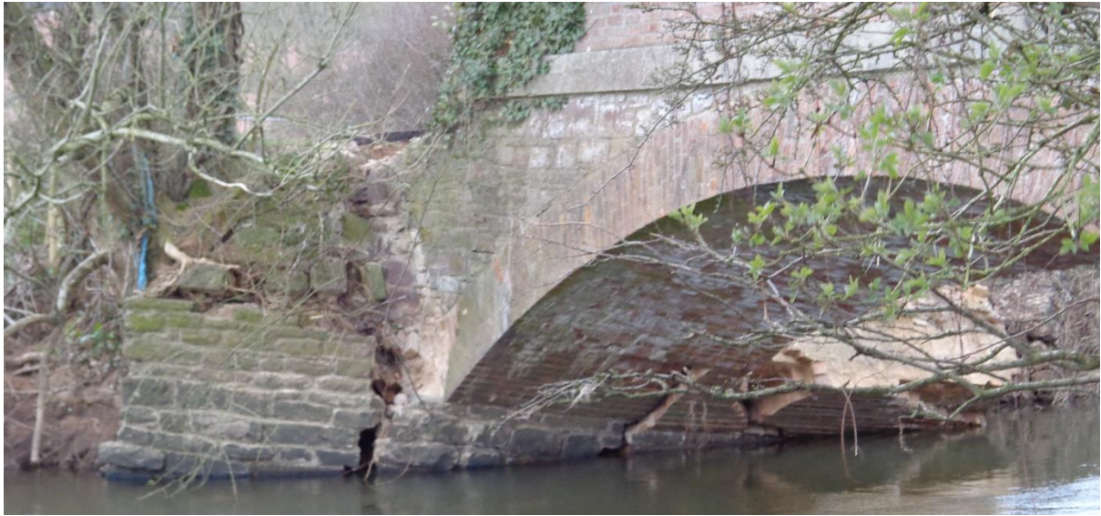
This view shows more. The abutment has completely broken up. Poor bridge didn't stand a chance.
