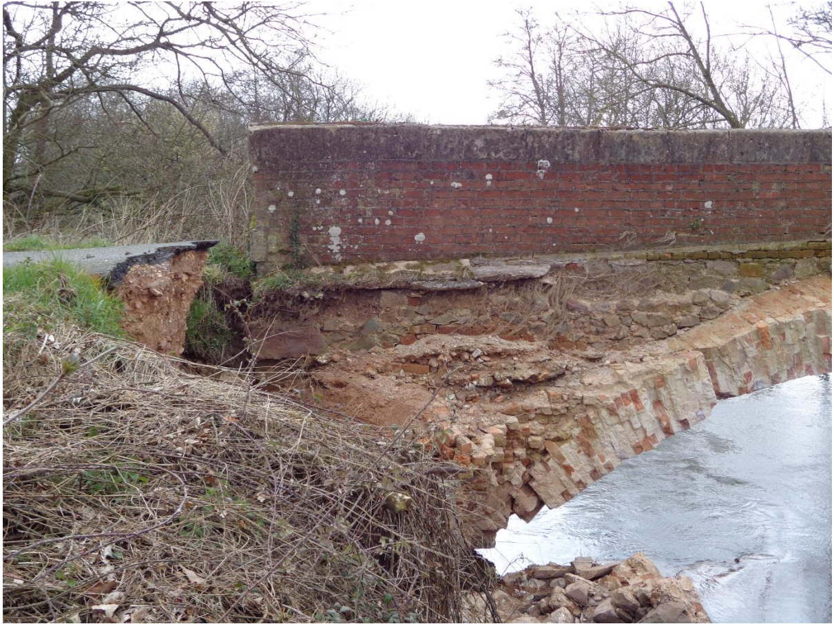
A more general picture shows that this abutment, too, has dropped considerably. Look at the surfacing levels.
