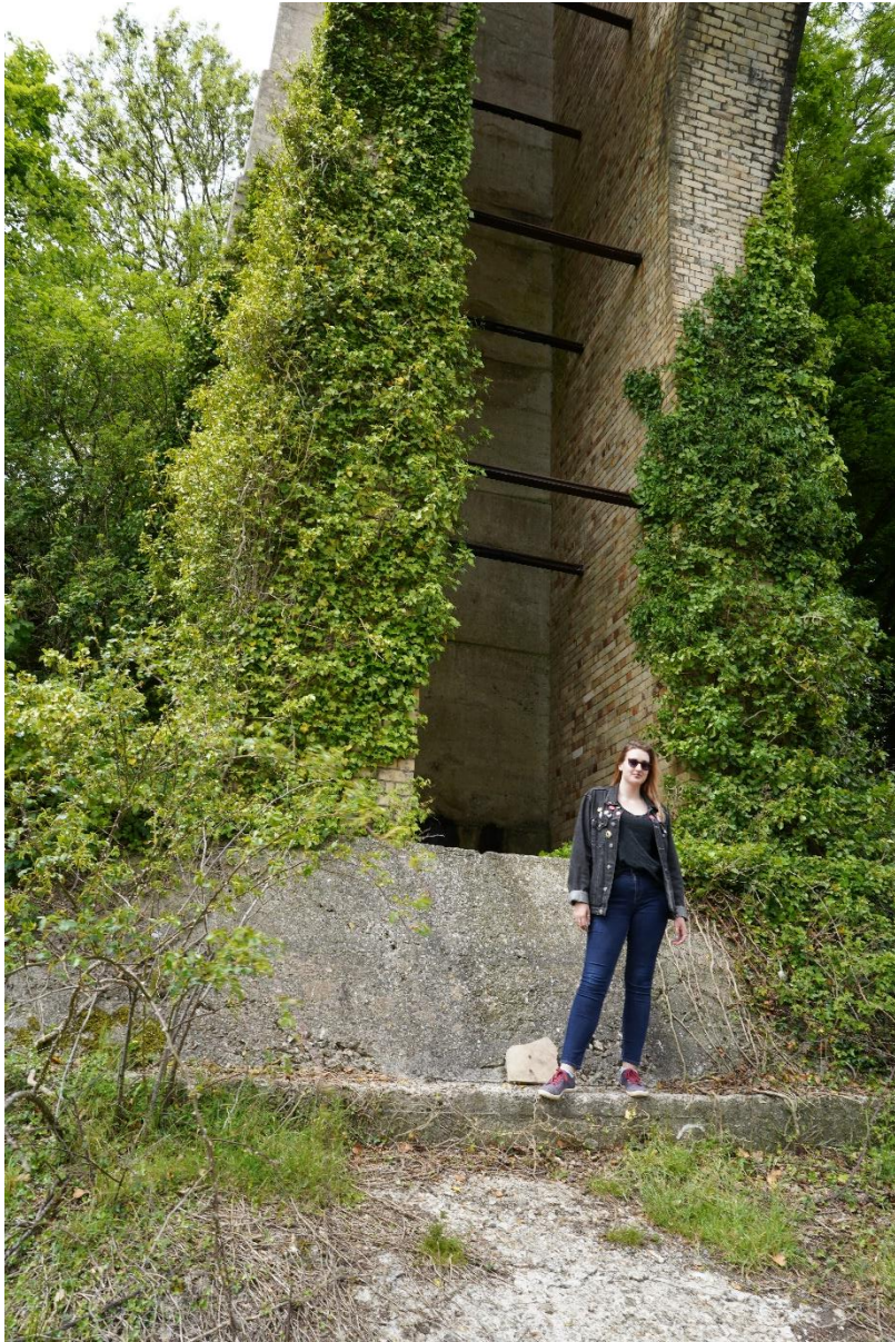
Here we have Bel to give scale to the construction. The concrete plinth here is an addition, as is the concrete surface on the valley side providing a prop from the pier below.
