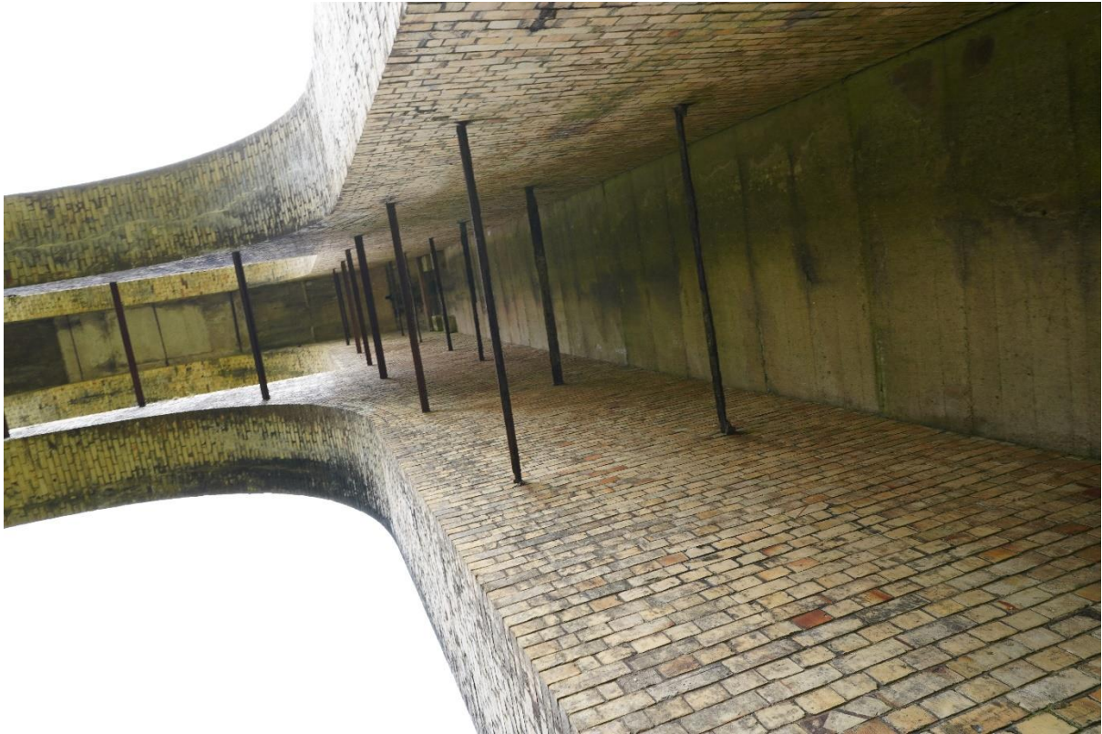
Looking up, the two brick sections are tied across with light gauge rail, much of which is rusting away.
