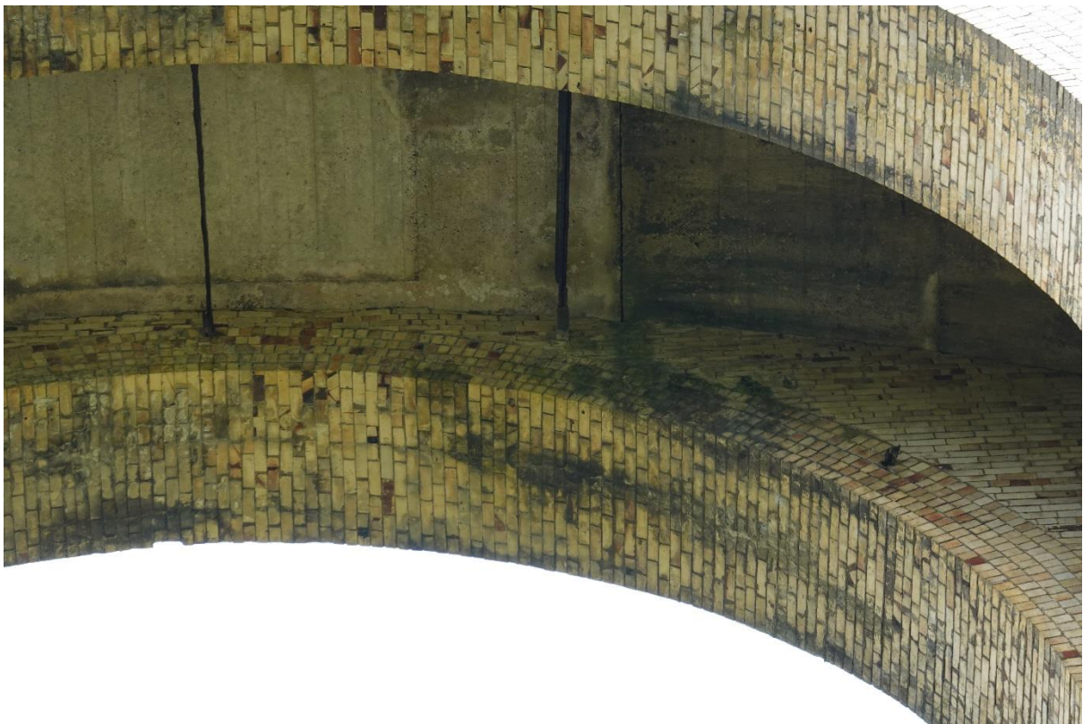
There is a hinge in the concrete arch at a construction joint. The articulation here suggests that the full height pier to the right has settled more than that to the left, which raises questions about
