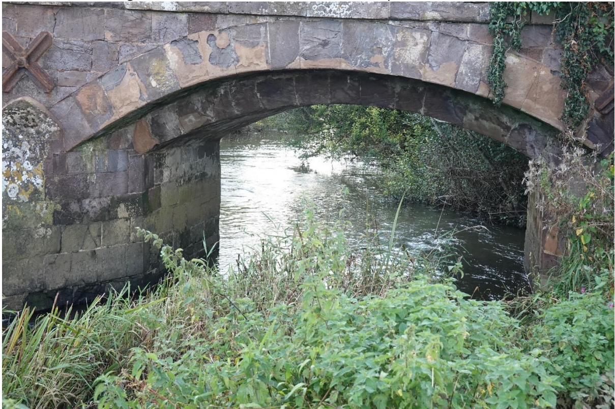
A definite sag in the string course, so these widenings dropped when the centring came out.
