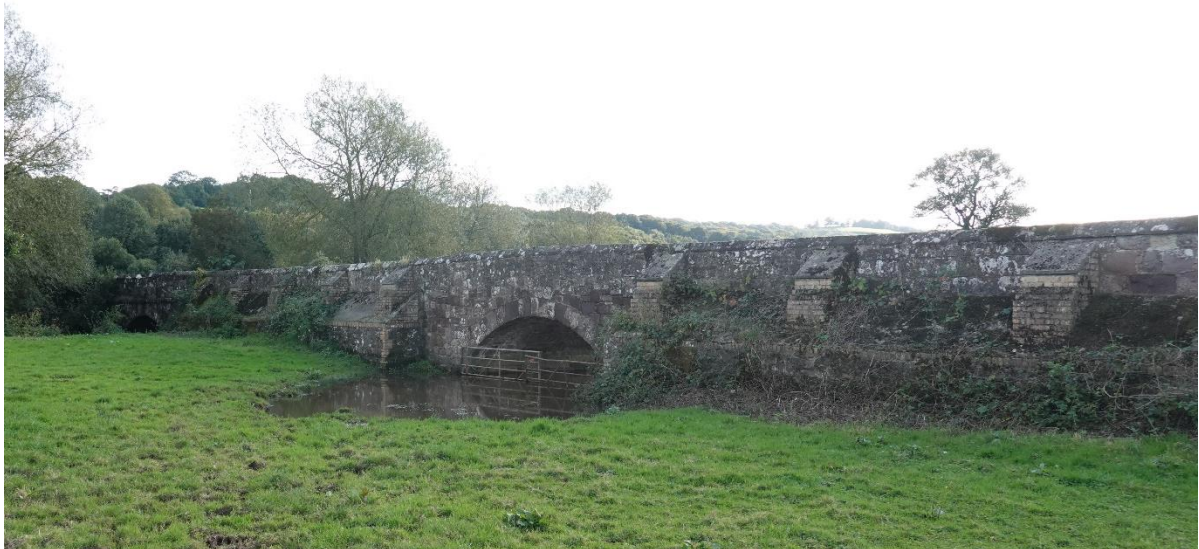
As at Clyst St Mary, the walls are tilting somewhat. Because this road is well trafficked, buttresses have been added.
