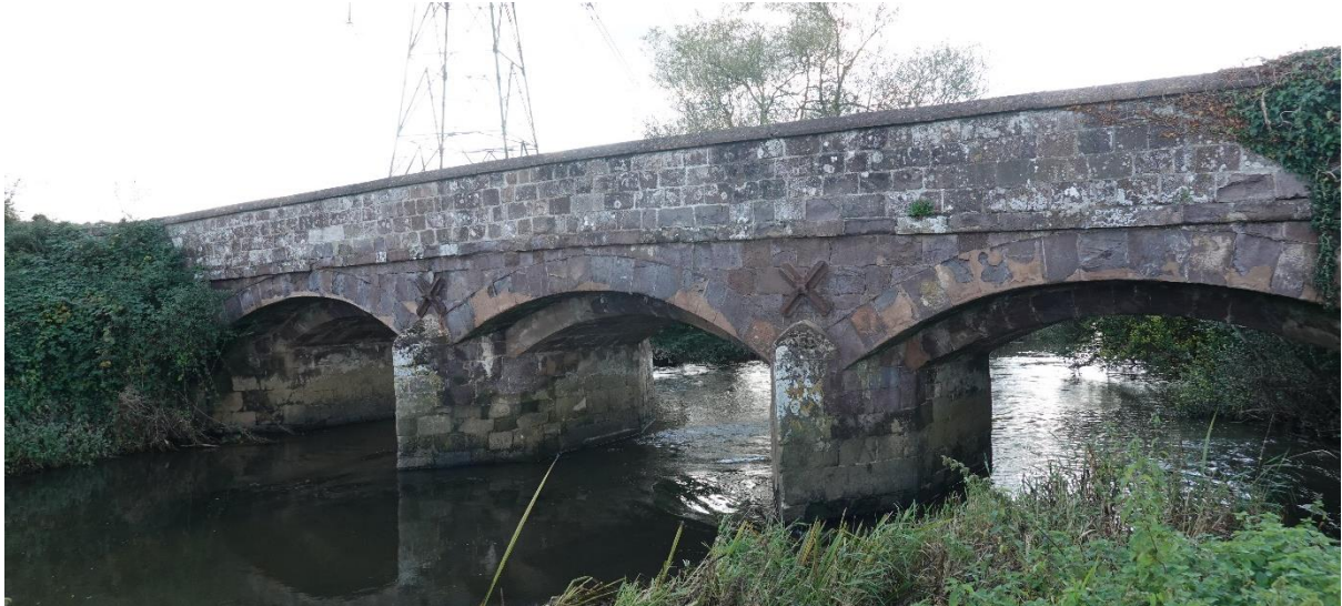
Here is the river bridge from the north east. Even on the multi spans, the arches are flat.
