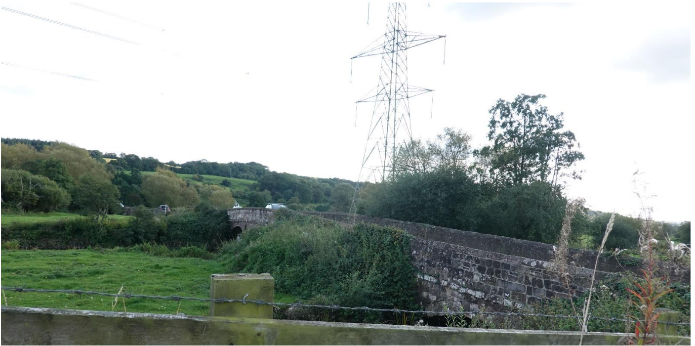
Here is a view from the east/south with the causeway stretching beyond the trees with a car just appearing.
