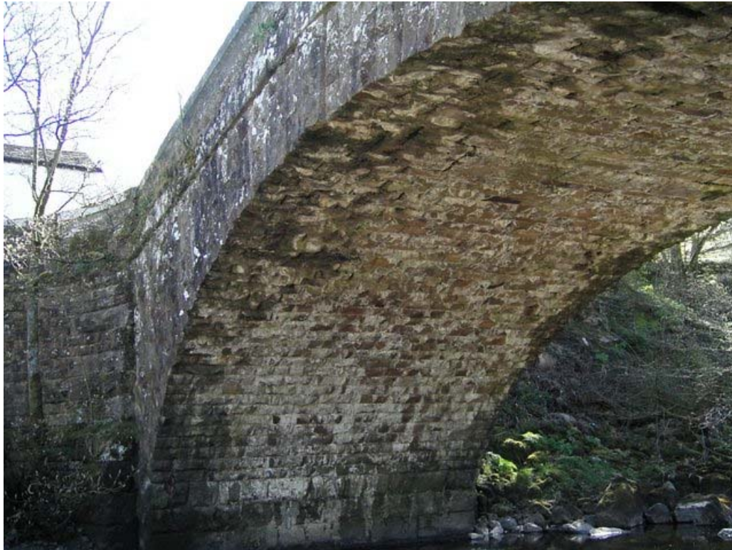
The soffit shows a change in colouring at what must be the top of the backing.
