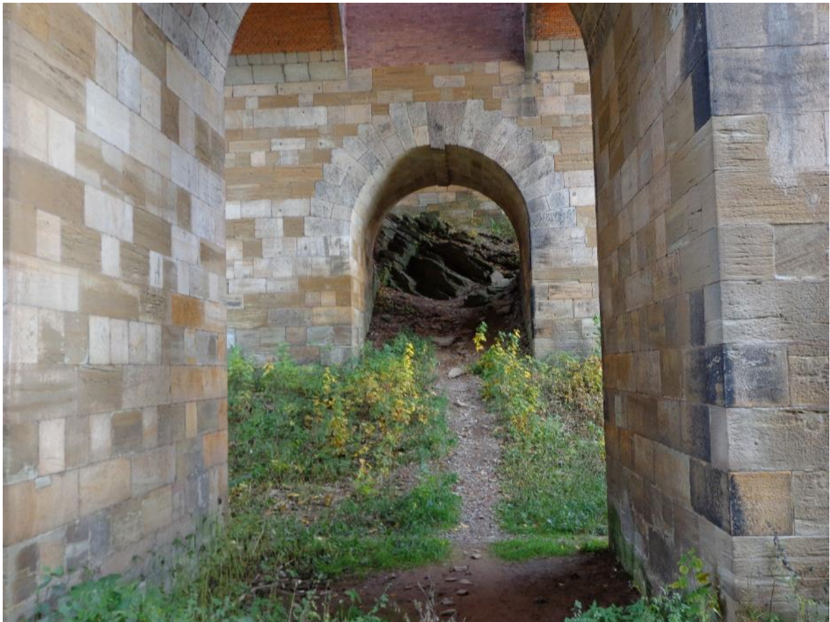
The whole viaduct begins with a stone plinth. This view along the lowest cross arch shows how the rock might dip steeply towards the river making foundations more difficult.
