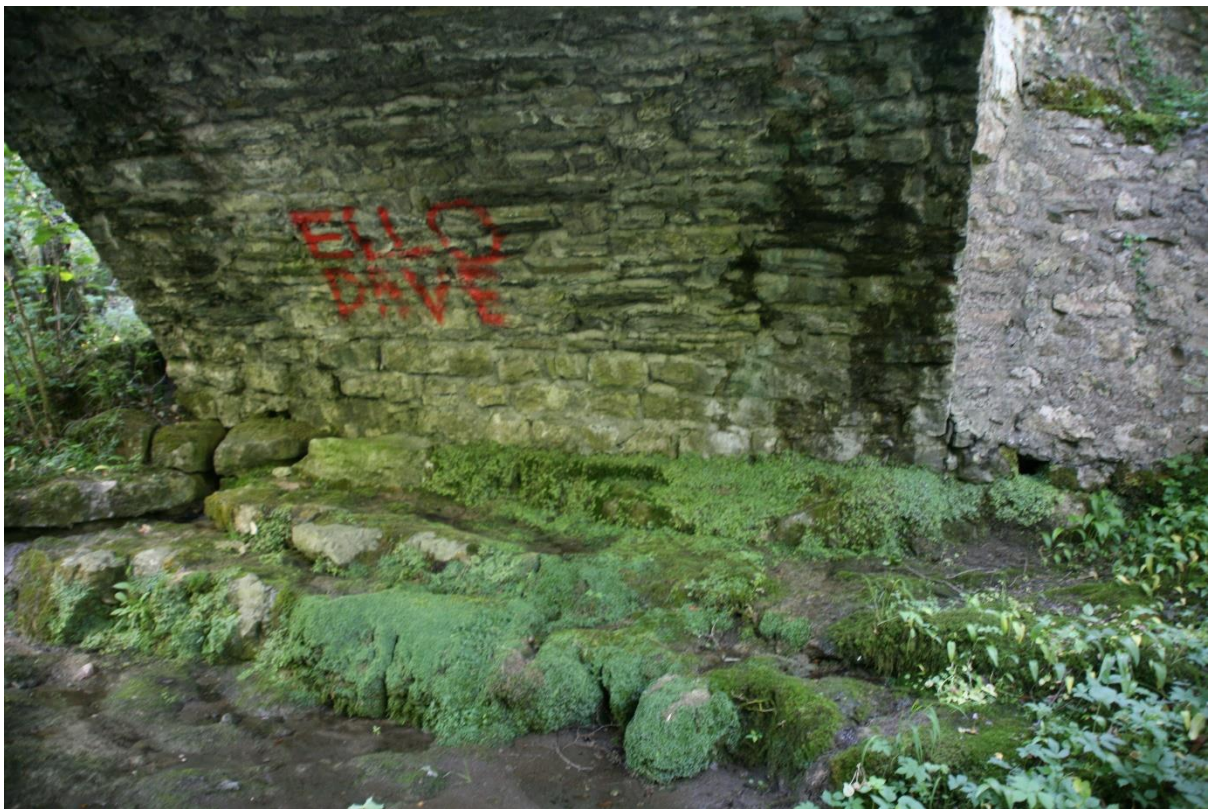
The downstream side arch is built from slatey material selected rather than cut and laid, in places. At odd angles. The pier is widened as a solid piece and one wonders whether the widening and the construction (or reconstruction) of the side span were done together.
