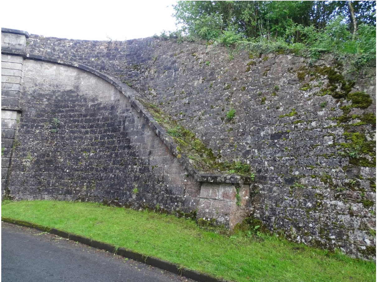
The arch has a substantial skew. This photo also shows the batter on the buttresses.
