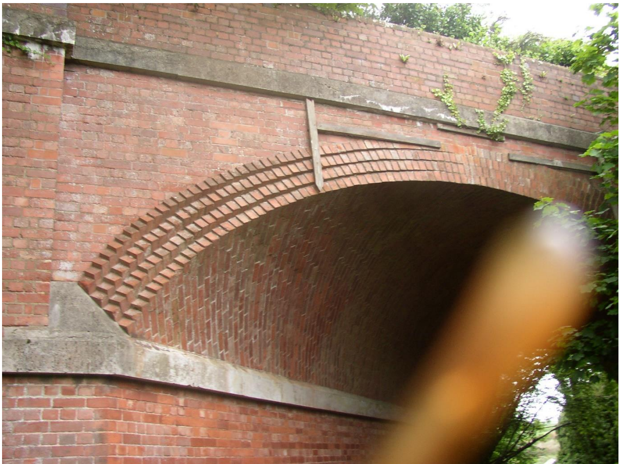
And this one in Exeter, where the brick ends are cut off to fit.
