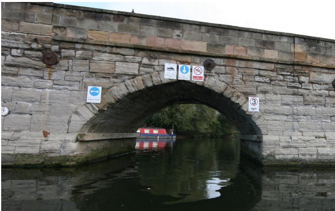
He boaters obviously find the upstream passage much easier. No impact damage on the edges here, though the span itself is similarly eroded.
