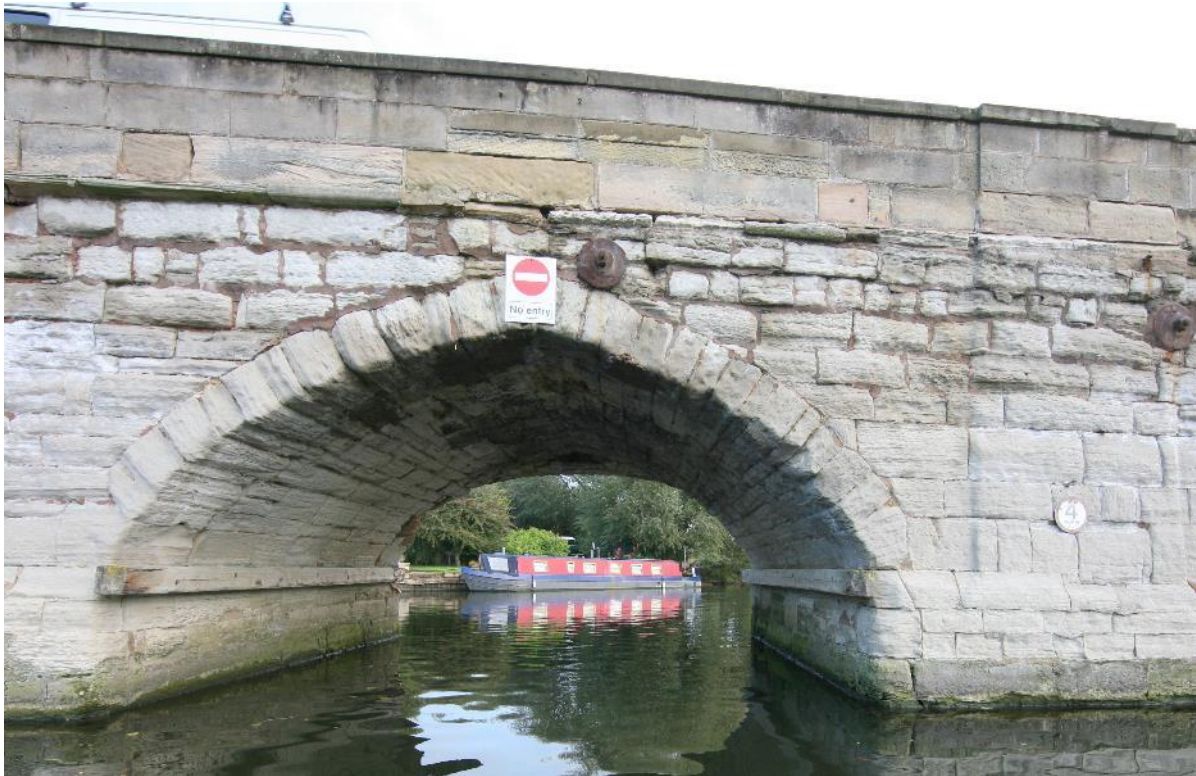
The view from downstream shows that the widening arch actually drops below the original at the crown. This is the only span in which this is true.
