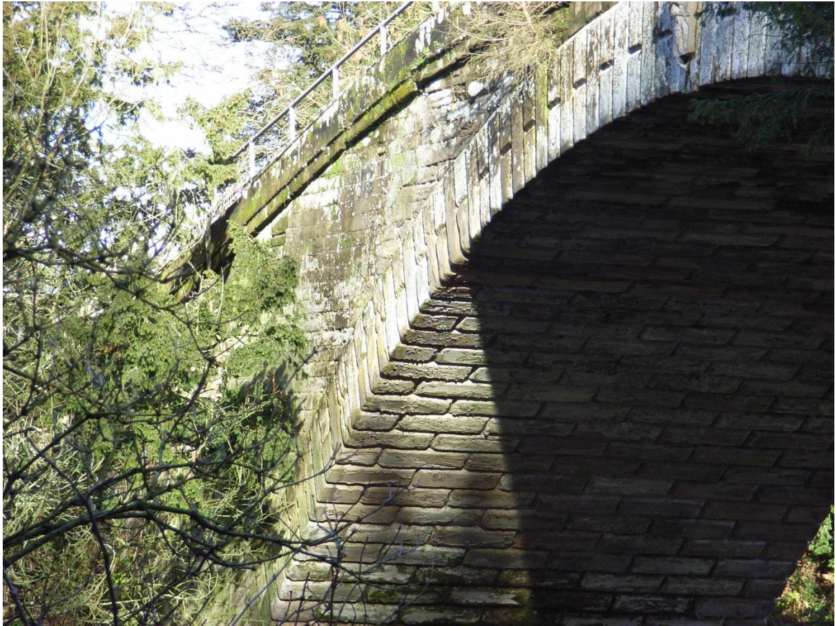
General weathering of the stone is visible here
