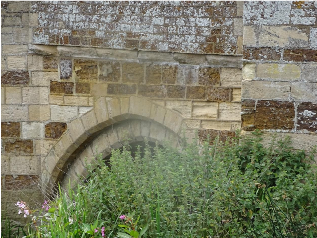
Here is more chemical weathering and a small (but badly weathered) corbel under the parapet.
