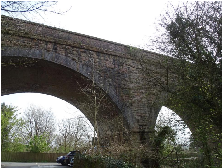
This view of the north side shows no drains either but it does show dark staining below what is presumably a more or less waterproof layer through the bridge.
