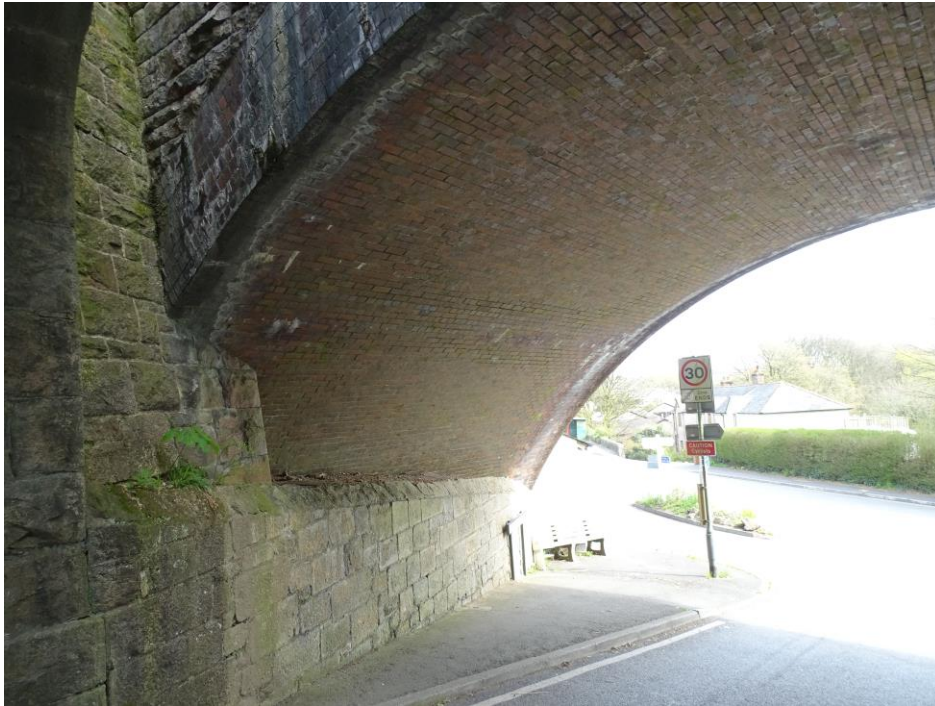
This oblique shot from below shows bands of brickwork with solid and eroded mortar. The erosion almost certainly corresponds to areas where there is water penetration from behind.
