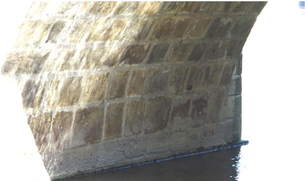
The coursing at bottom right in this photo is definitely not true, suggesting that there has been some serious erosion at some point.
