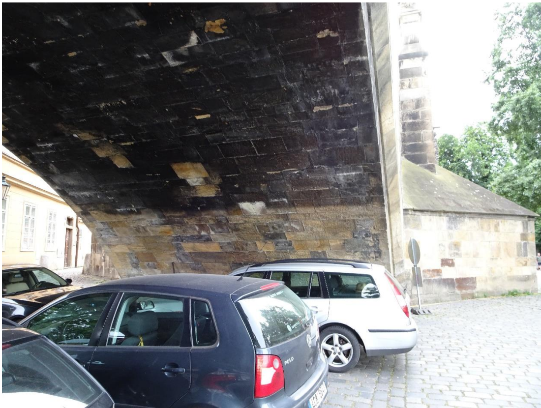
And is this fire damage under the land span? Certainly a car park seems a sad use for such a magnificent bridge.
