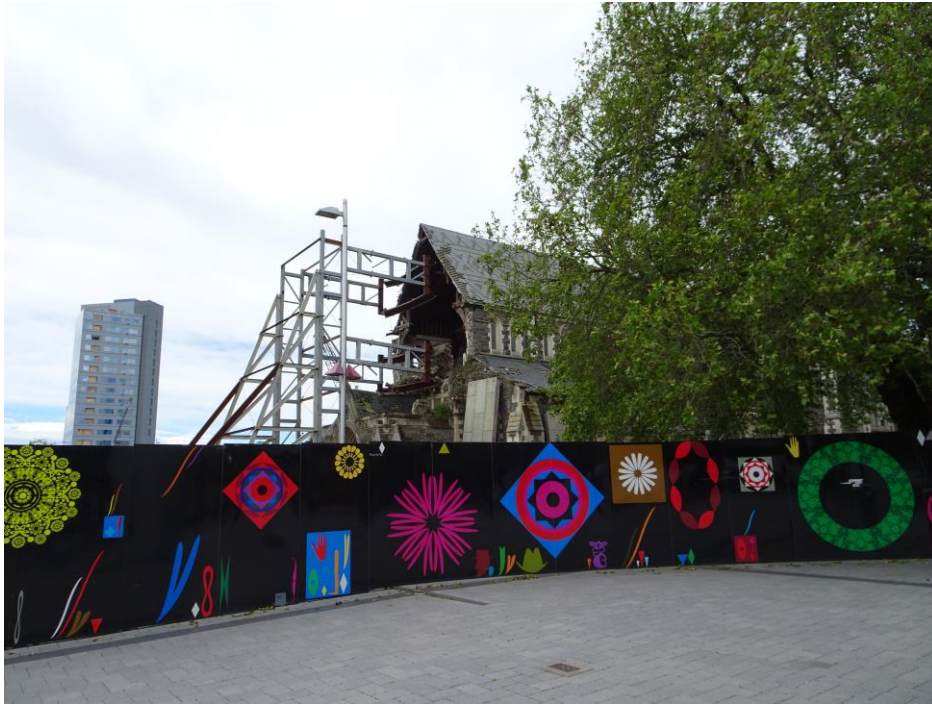
Note the bent steelwork here where walls have fallen despite the attempt to support them.
