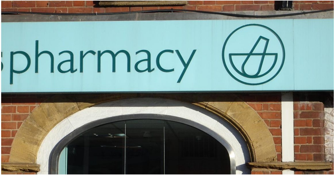
Notice the crack just peeping out to the left of centre. Some movement going on here.
