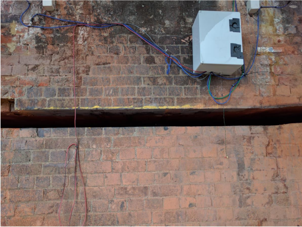
Vertical deflection gauge mounted in enclosure, with wire across gap.
