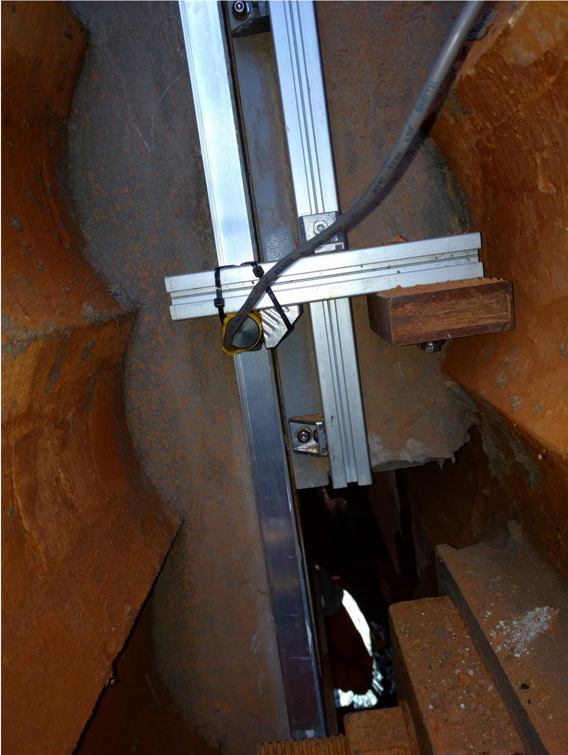
Transverse movement gauge mounted on sliding bearing.
