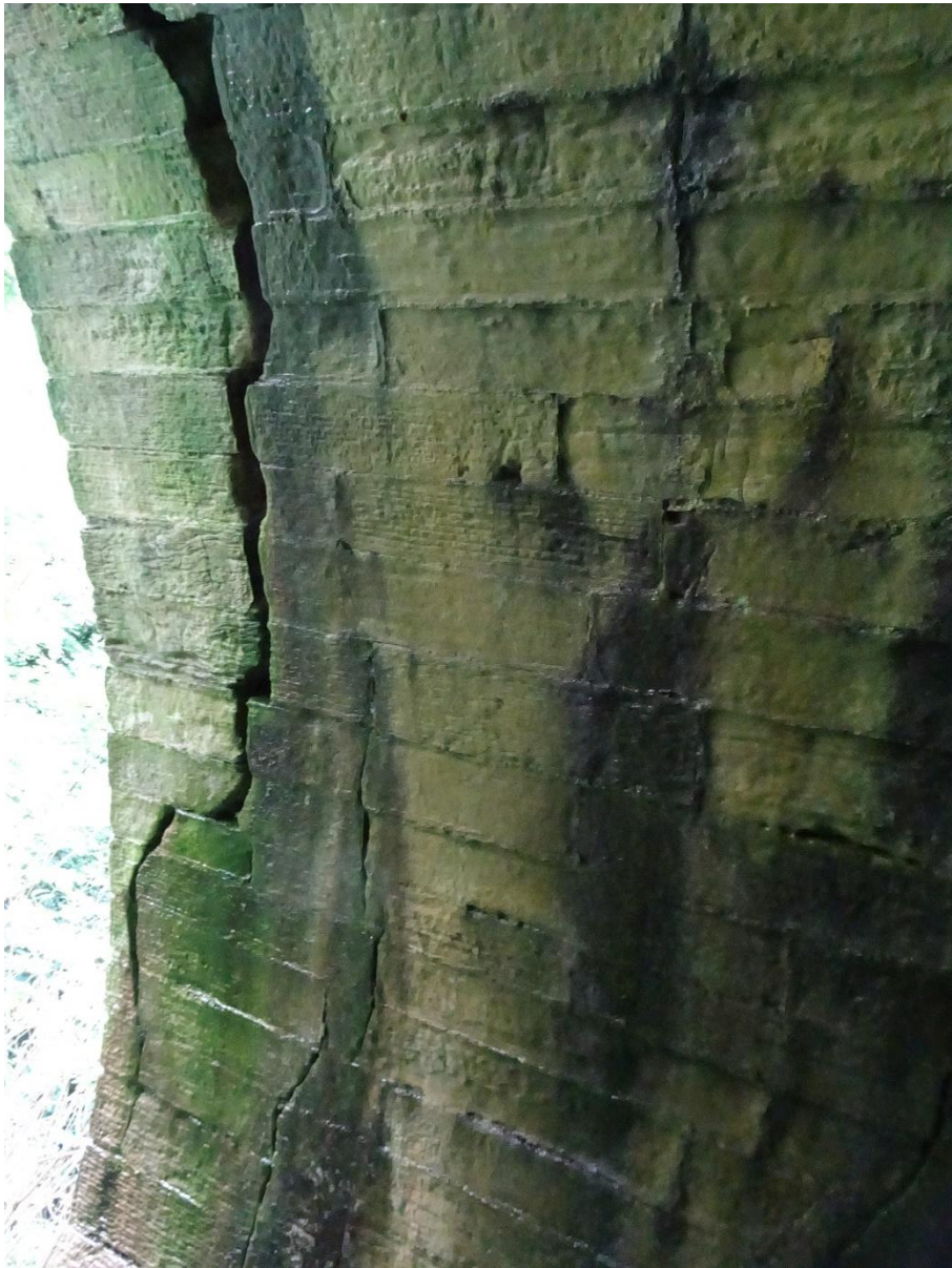
This is the “good” end of the crack.
