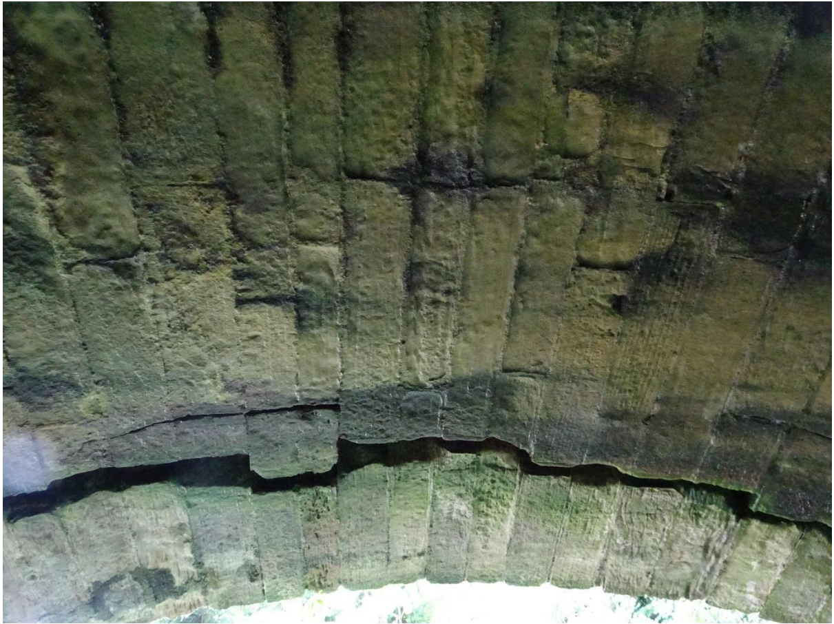
Here is the damage at the crown.
