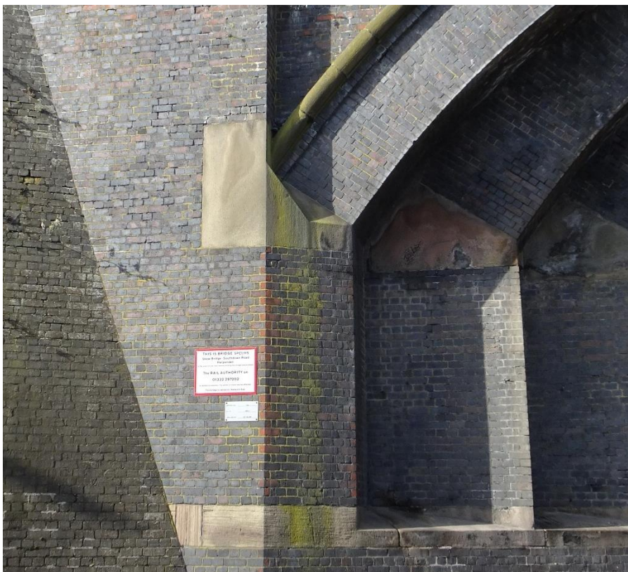
The end skewback is a magnificent piece of masonry work. The original piece of stone must have been a metre high and wide and nearly 2m long.
