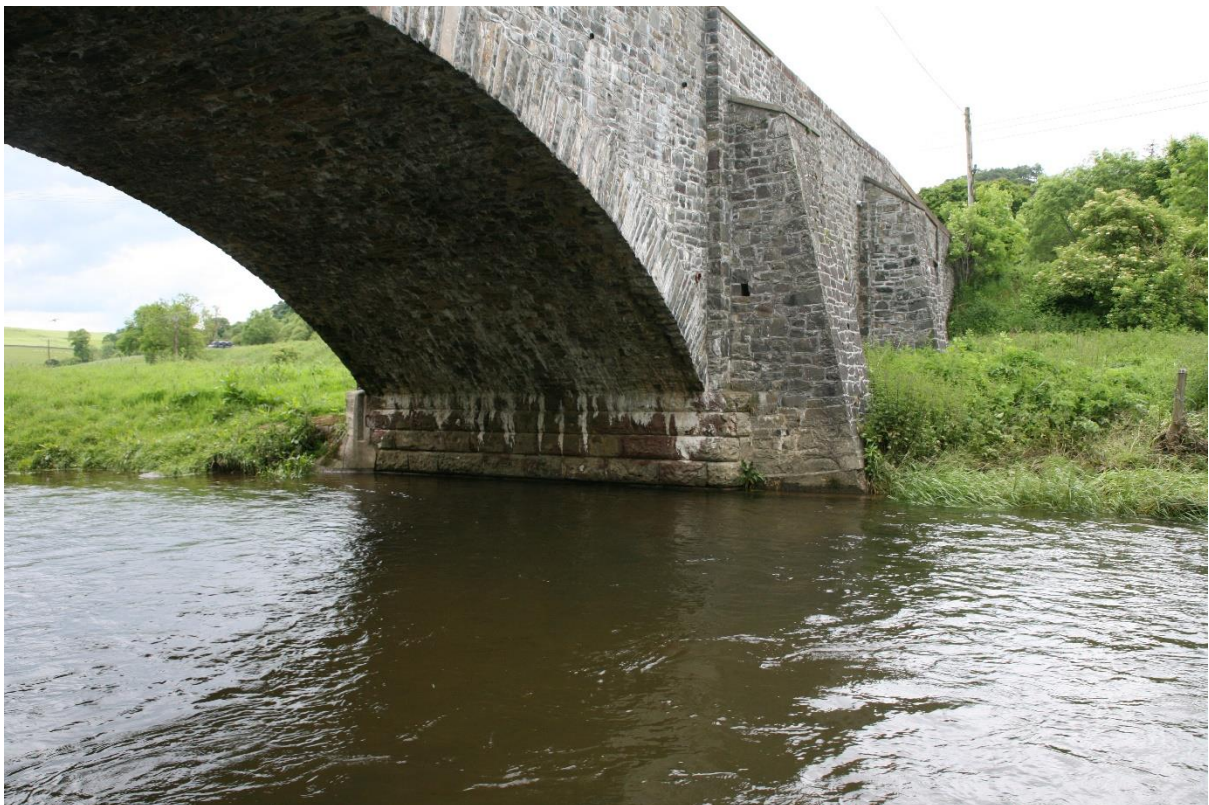
This shot from below barely shows the soffit but provides an opportunity to shout out for Affinity Photo which has amazing powers of enhancement. See below achieved in three keystrokes.
