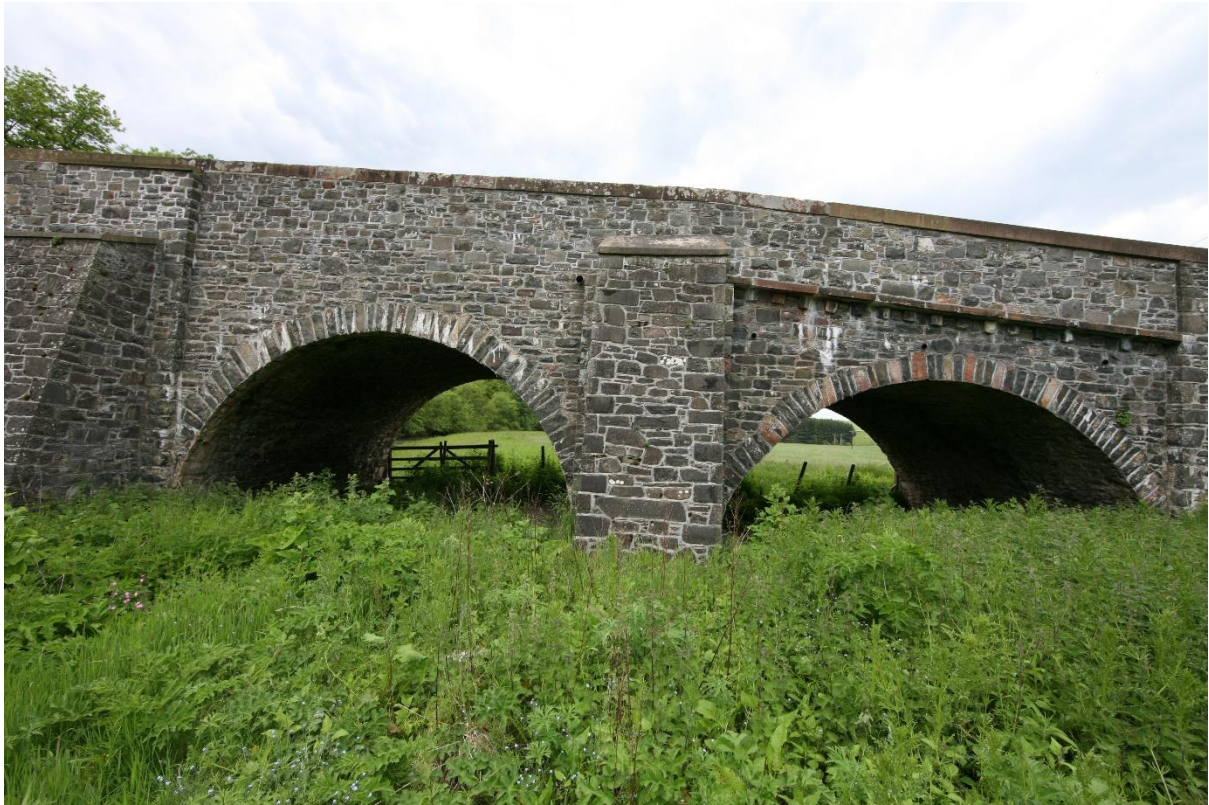
The side spans, or strictly flood spans, are interesting for being different radii, partly to accommodate the sloping road.
