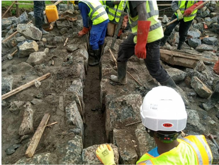
A layer of mortar over the centre in the bottom of the slot awaiting the final stones.
